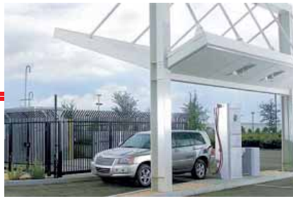
Hydrogen fueling station.
